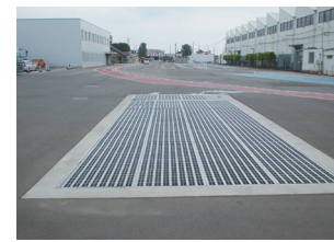
Flood prevention measure (drainage grid) (Utsunomiya Plant)
